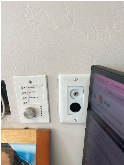
Pro Shop Wall Plate Controller and Audio Inputs
